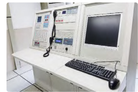
Third-party docking (fire fighting/CCTV)
